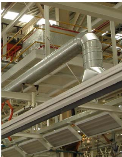
Slotted Suction Channel
