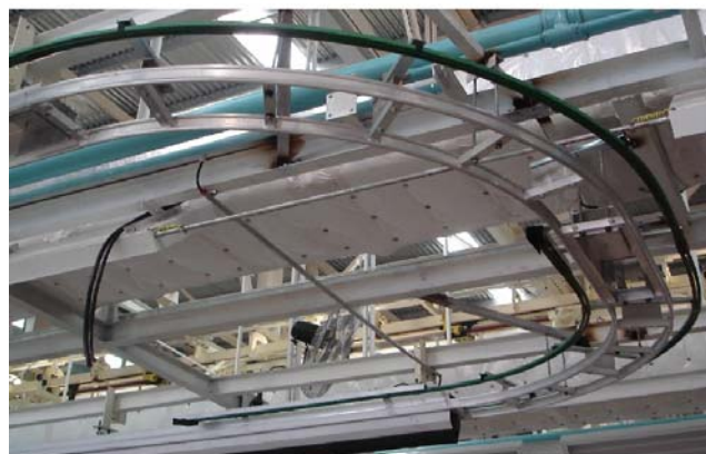
Exhaust Extraction System on a Final Assembly Line
